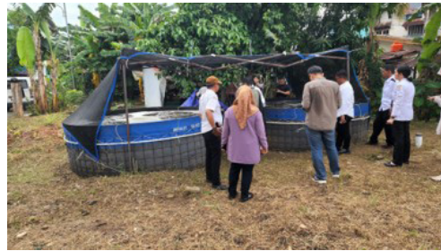
A team of NSF researchers traveled to Makassar to support the installation of solar panels in three of the garden alleys to power aquaponics and fish farms. Makassar, Indonesia (May 2024)
